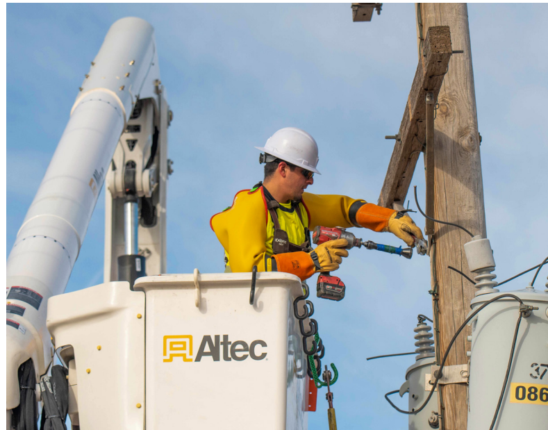
Crew Foreman Jacob Mendoza removes infrastructure from a pole to prepare it for replacement.
